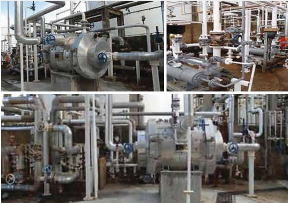
INSTALLATION NEW HEAT EXCHANGER E1601 COMPLETE WITH PIPING AND ACCESSORIES AT VCMSB
