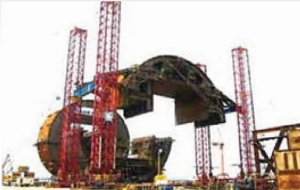
SUPPLY AND OPERATE 3200 TONS PUSH UP
