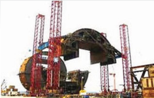
SUPPLY AND OPERATE 3200 TONS PUSH UP
